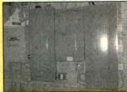
HOME EMERGENCY PANEL
